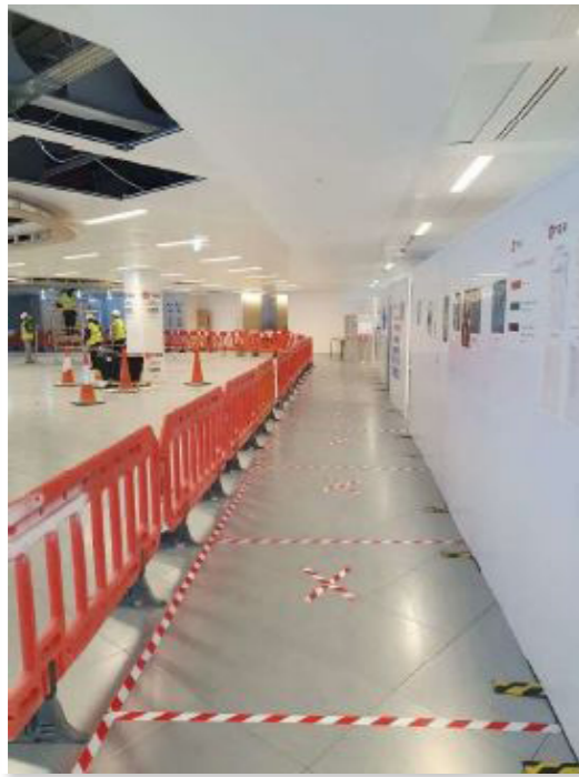
Floor markings in safe route on a one way system to site welfare to facilitate social distancing.
